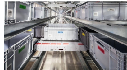
Reciprocating transport systems
