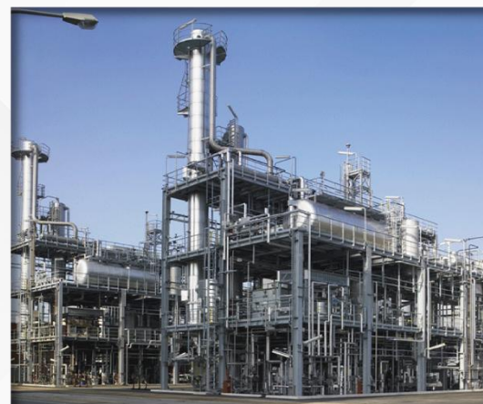
Fire Fighting Pipeline of Moroccan Chemical Plant
