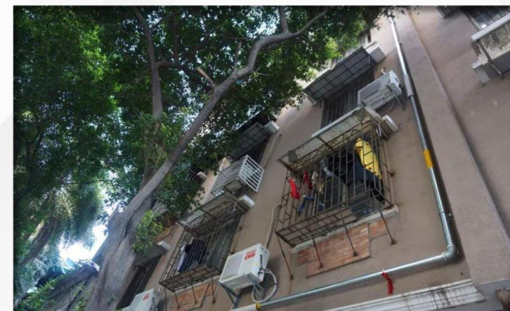
Galvanized steel pipe of Bolivia Civil Gas Pipeline
