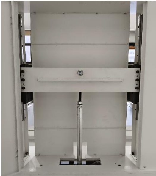
Main beam lifting guide rail
