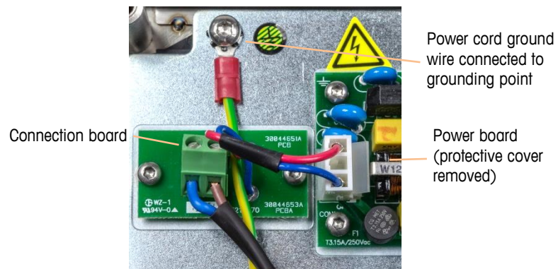
Figure 2-18: IND236 AC Power Connection Board and Grounding
